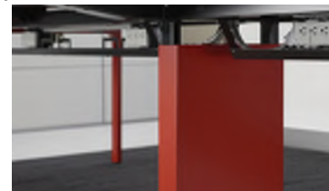
System Power Below
