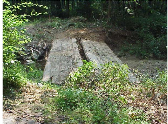
Figure M6.1: Poor vehicle access.
