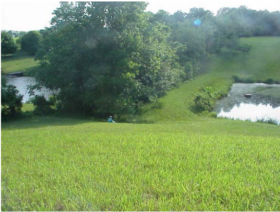
Figure 1.8: Woody vegetation on embankment
