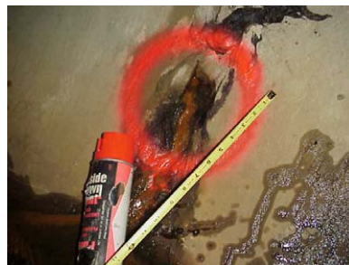
Figure M3.4: Rust intrusion demonstrates improper pipe joint.
