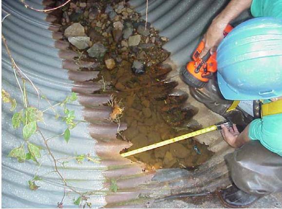
Figure 1.4: Pipe invert abrasion
