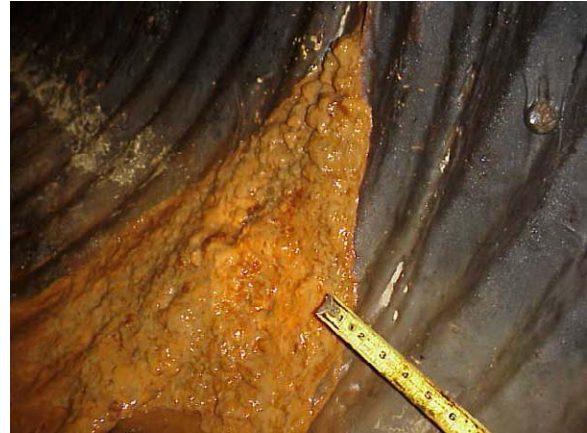
Figure M3.2: Soil entering open pipe joint.
