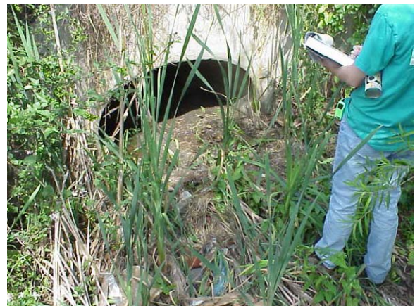
Figure M4.2: Excessive vegetation near an outfall.
