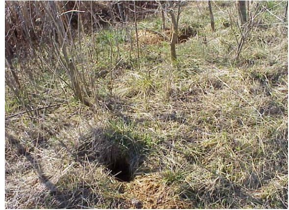
Figure 1.17: Animal burrow in pond embankment.
