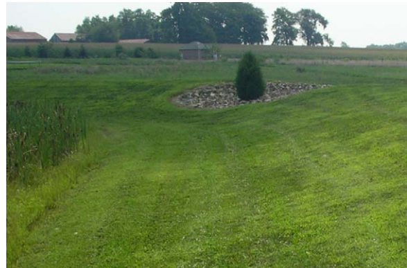
Figure M4.5: Unwanted vegetation - tree on embankment.
