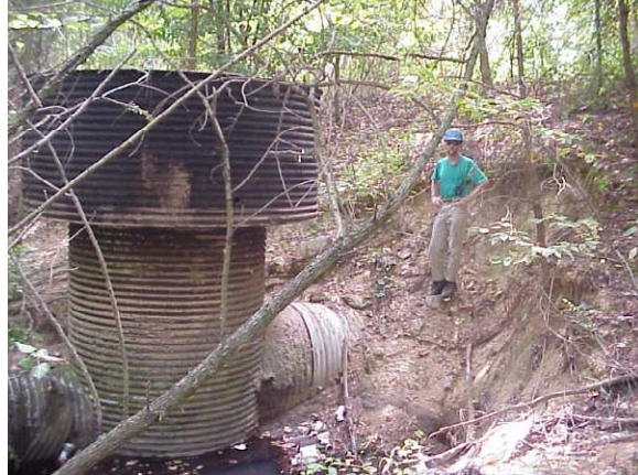
Figure 1.5: Severe erosion around riser and barrel
