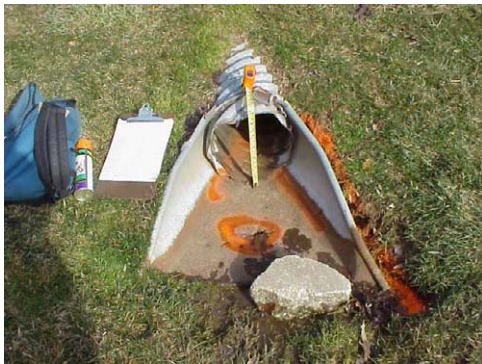
Figure 2.1: Marking outfall deficiencies.
