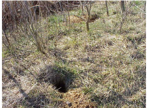
Figure M8.1: Animal burrow in pond embankment.
