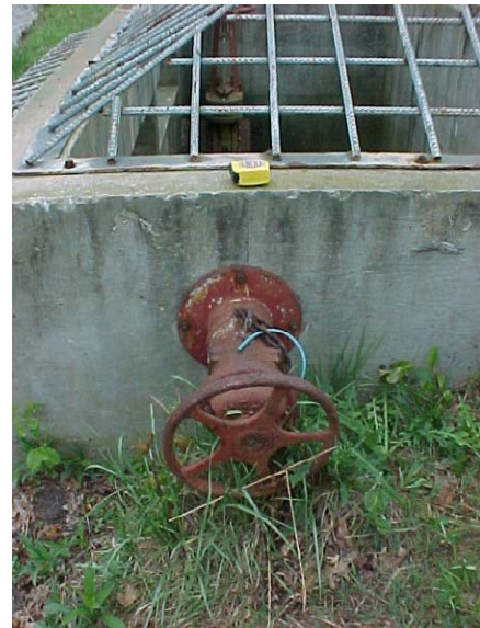
Figure M7.1: Valve outside riser.
